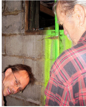
Steve Maki and Mel Kaehler work on the water heater. Having fun, Steve?
